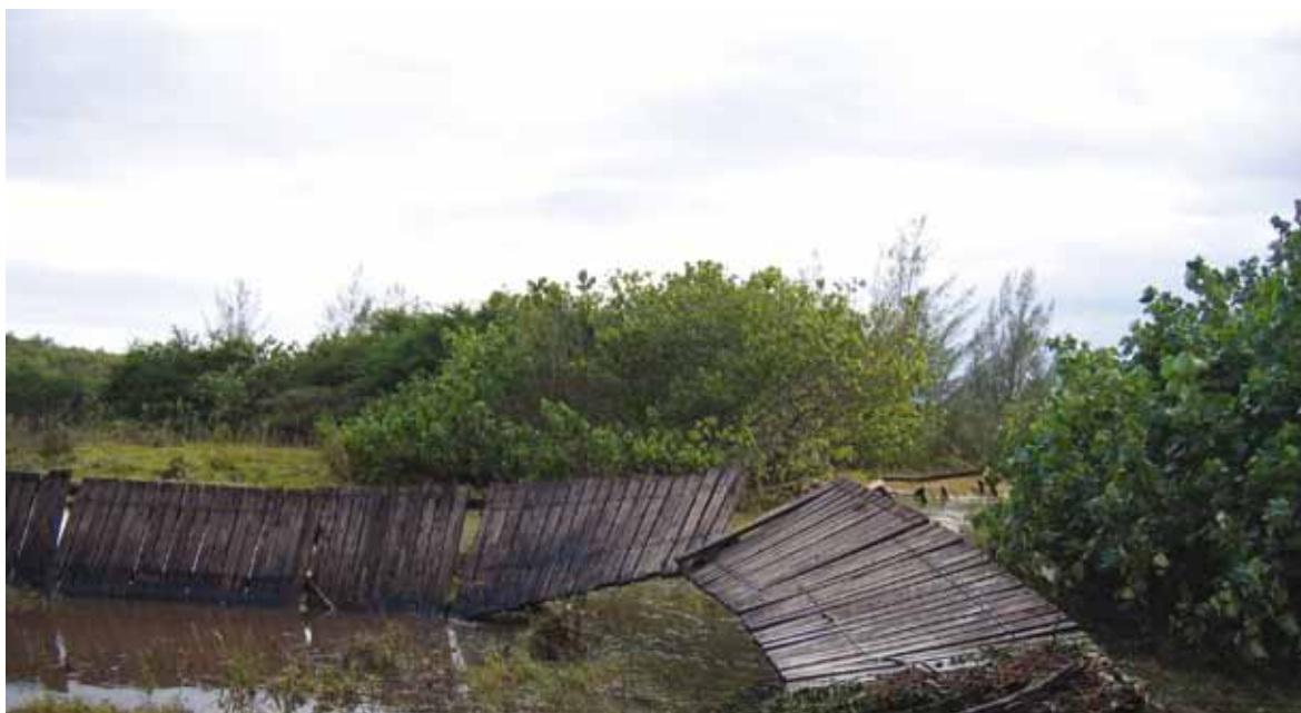
Fig 7: Cyclone Gamede's high seas damaged the board walk on the northern estuary bank— a sharp reminder of the need to keep hard infrastructure to a minimum in this dynamic environment (photograph: iSimangaliso Authority).
