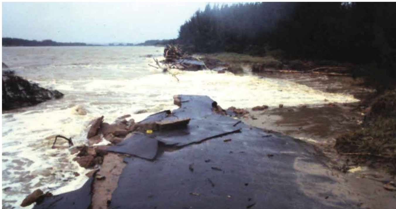
Figure 21: The cyclone Domoina floods and the associated high seas removed the concrete retaining wall, dolosse and road on the north bank at the mouth. (photograph: A. T. Forbes)
